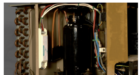
10 Check correct wiring & replace covers
